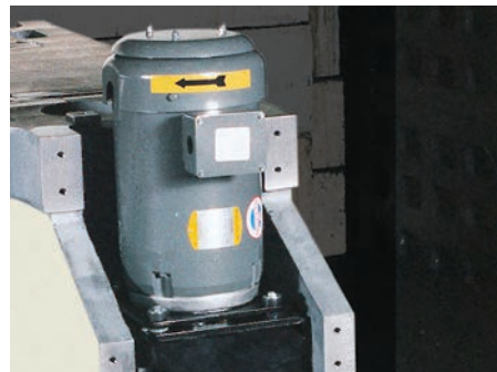
Hydraulic motor pump assembly mounted in left hand rear press bed leg.
